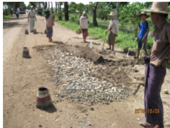
Figure 3: Damaged roadway after flooding
