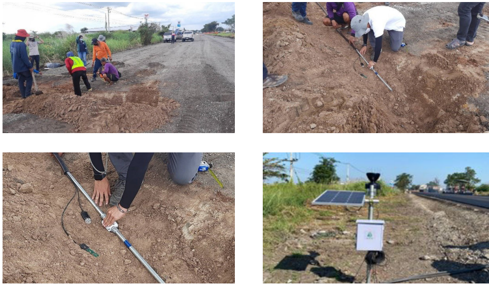
Figure 4: Installation of field monitoring instrument
