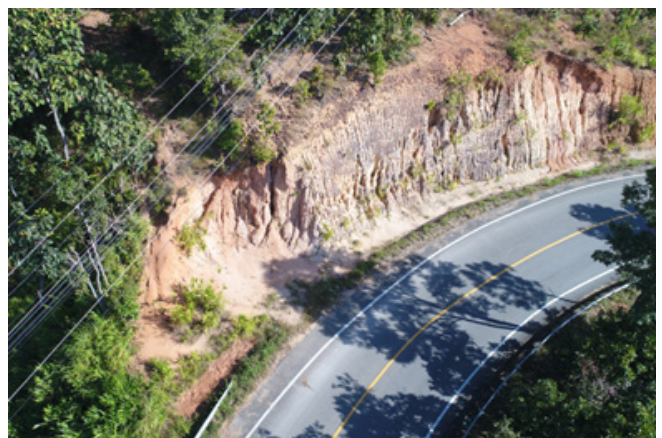
Figure 1: Slope erosion and failure at Highway No. 1192, Chiangmai Province
