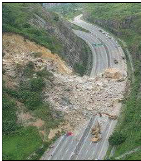
Figure 11.2: Typical problem related to slope stability in hilly terrain
