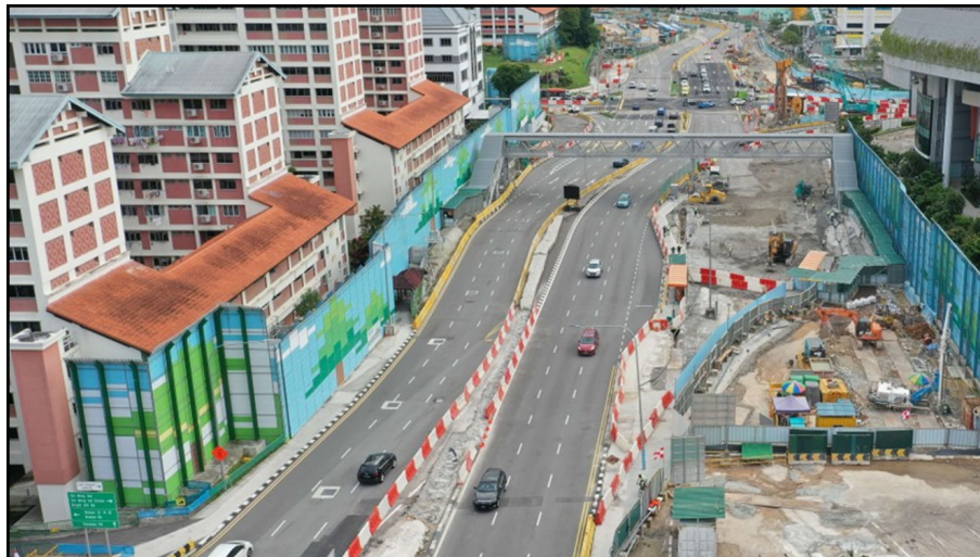
Perimeter noise barriers for noise management
