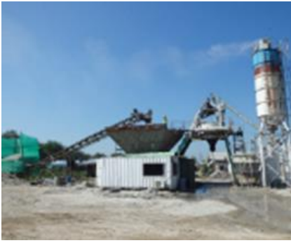
Figure 32: Local mixing plant
