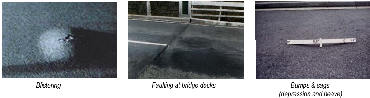
Figure 3-18: Typical distress types – flexible pavements (Sources: REAAA Indonesia, Korea, Japan: Austroads 2019b; NZTA 2001)
