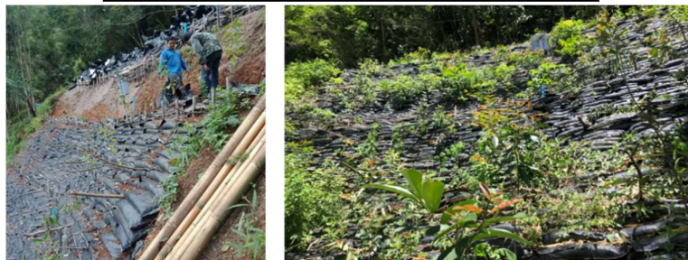
Figure 2: Bioengineered slope using screw-piles and vegetated flapped soil bags at rural road 4088, Kanchanaburi Province, Thailand
