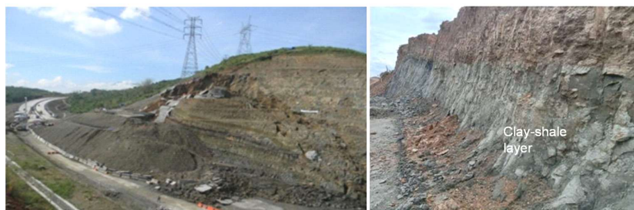
Figure 8: Slope failure at Toll Road Semarang-Bawen, Central Java, Indonesia
