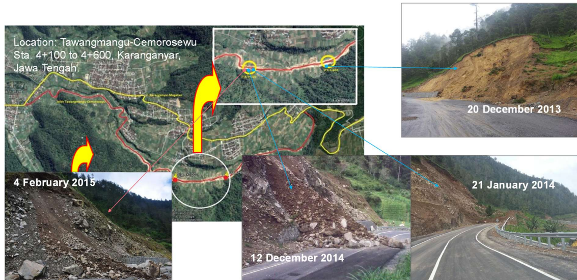
Figure 7: Debris deposit of the roadside slope failure: Tawangmangu-Cemorosewu road in Central Java
