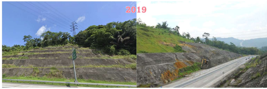
Figure 9: Slope remedial measures using shotcrete and bolt at Toll Road Semarang-Bawen: (left) successful work, (right) unsuccessful work
